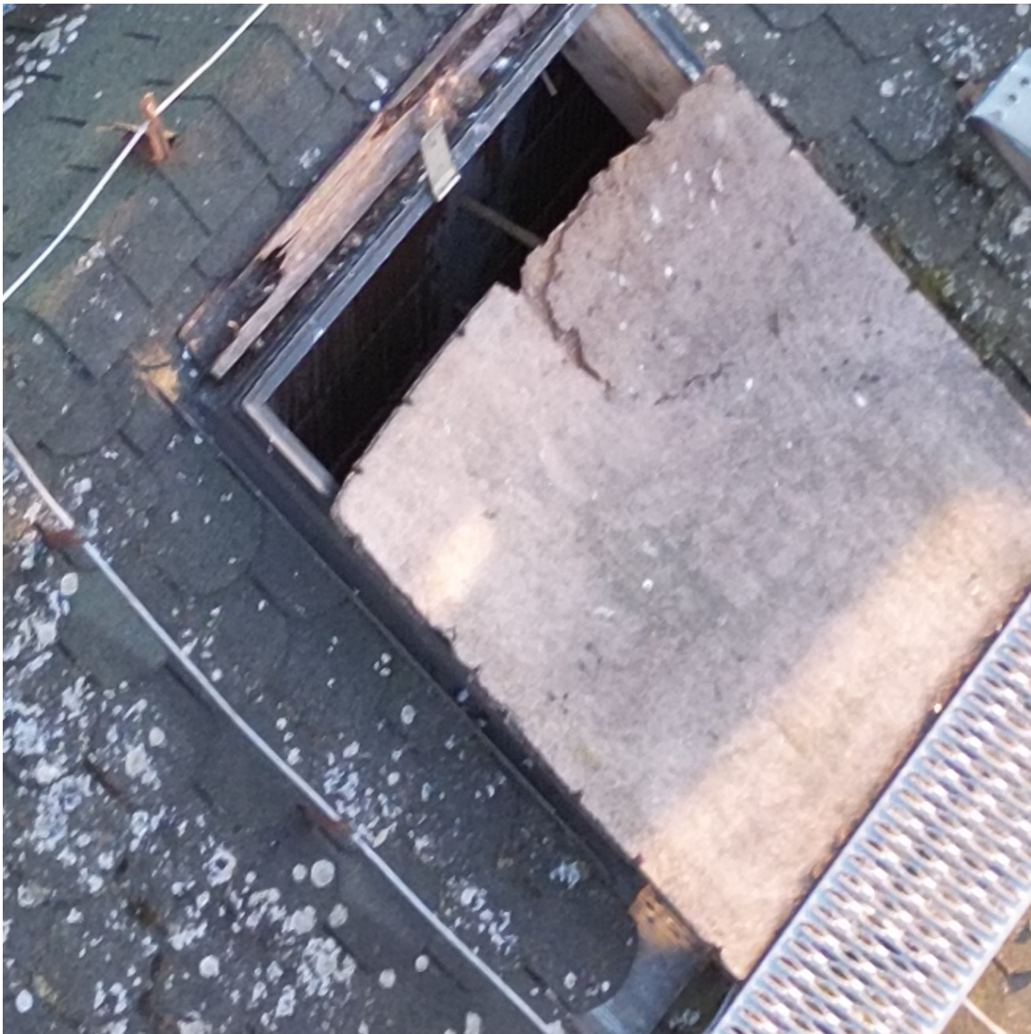
Photo 08. A rectangular opening with a panel partly over or beside it; urgent verification is required.
