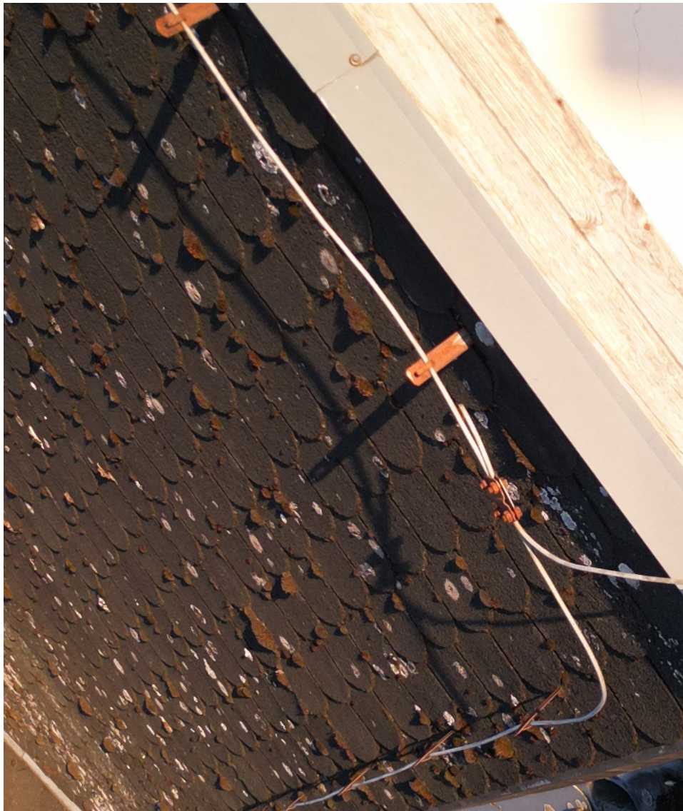
Photo 09. Material accumulated in the gutter and cables routed near the eaves.
