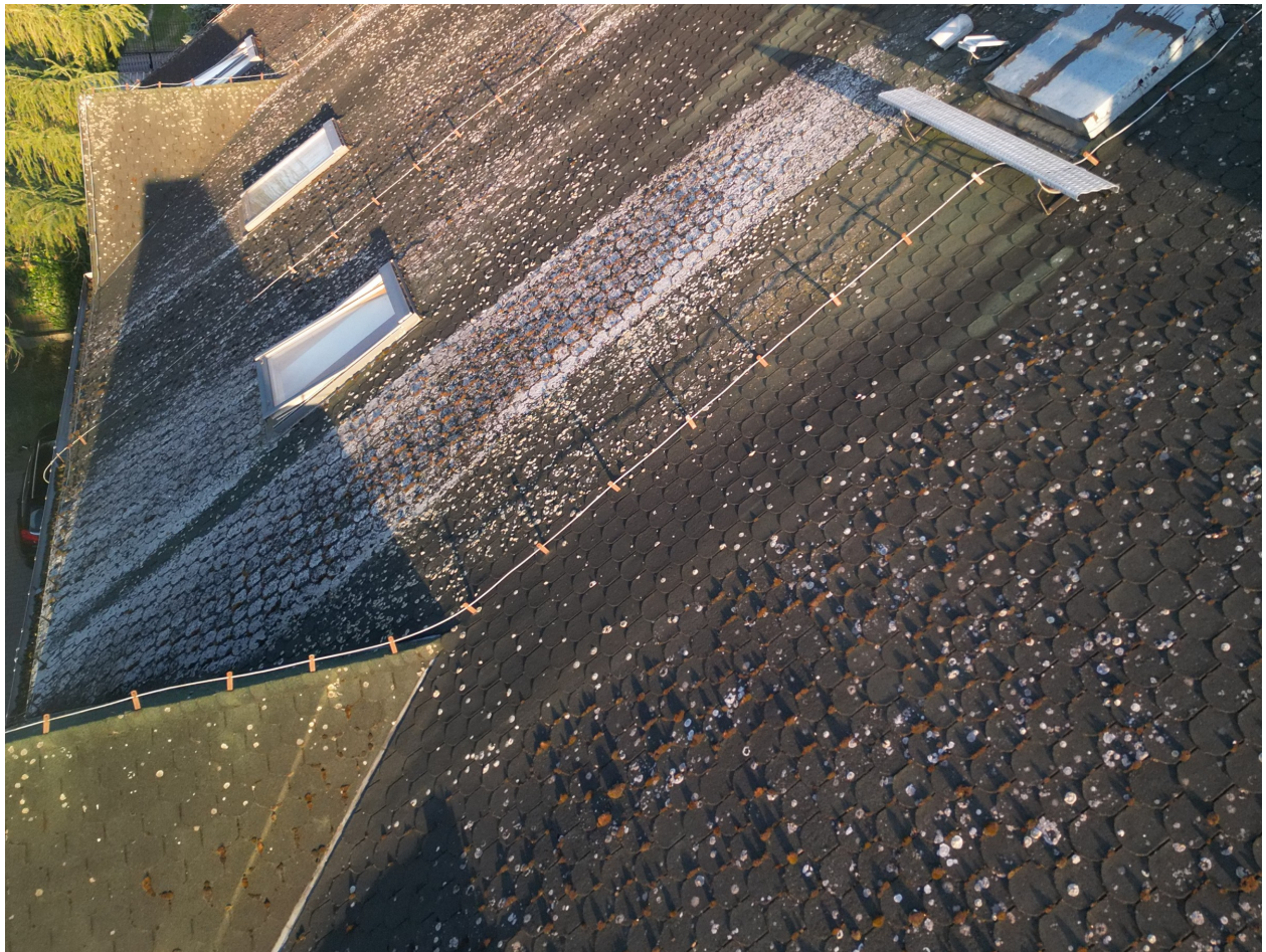
Photo 07. Extensive deposits and local variations in the appearance of the covering across several roof planes.
