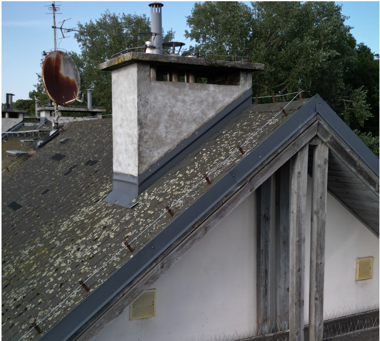
Photo 04. Extensive corrosion on one dish, deposits on the covering and chimney caps, and weathered timber.
