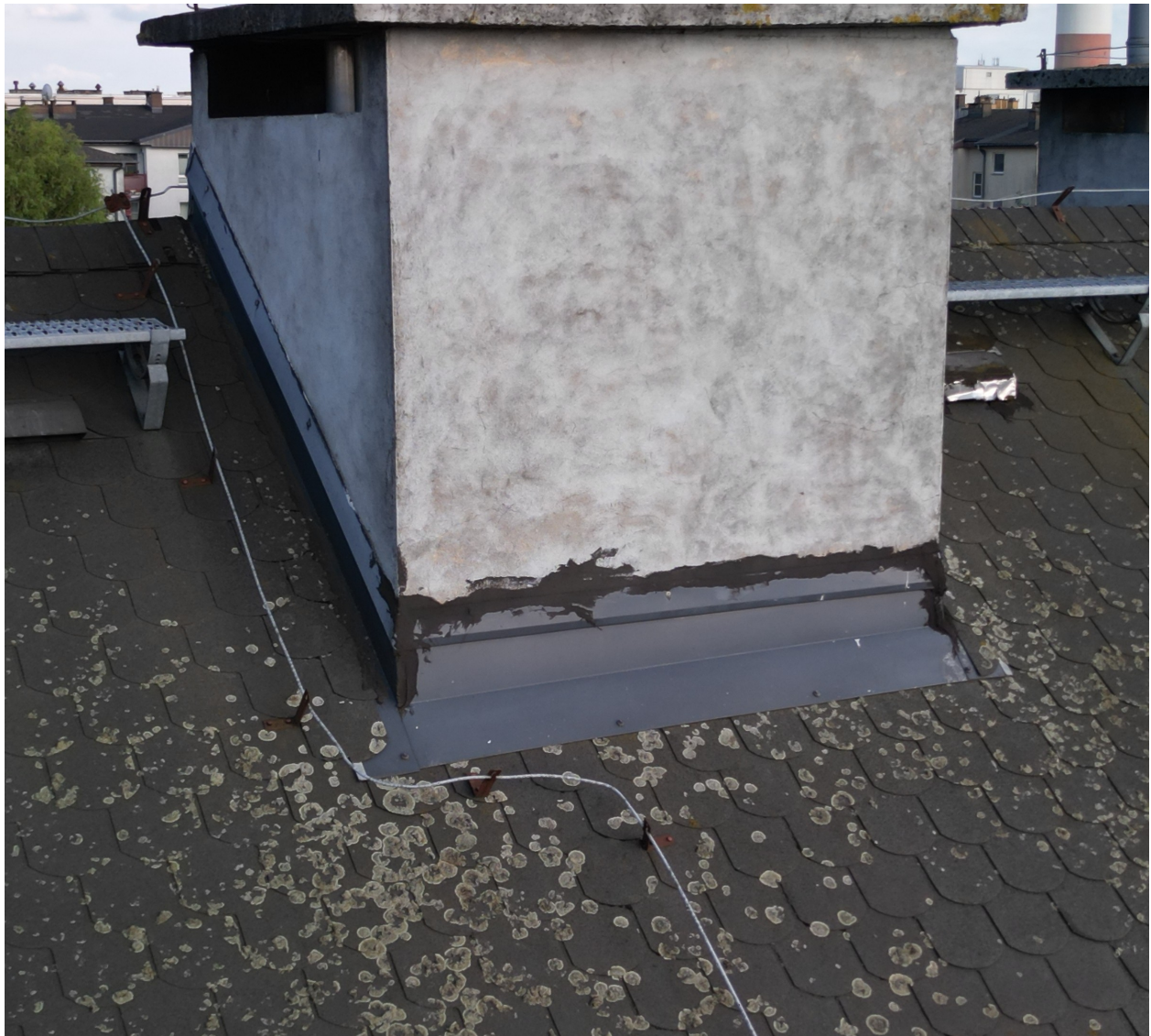
Photo 03. A strip of apparent repair or sealing material is visible at the chimney base, with deposits on the covering.
