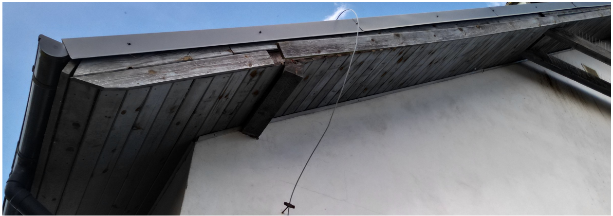
Photo 05. A local discontinuity in a timber board at the eaves and a loosely routed cable.
