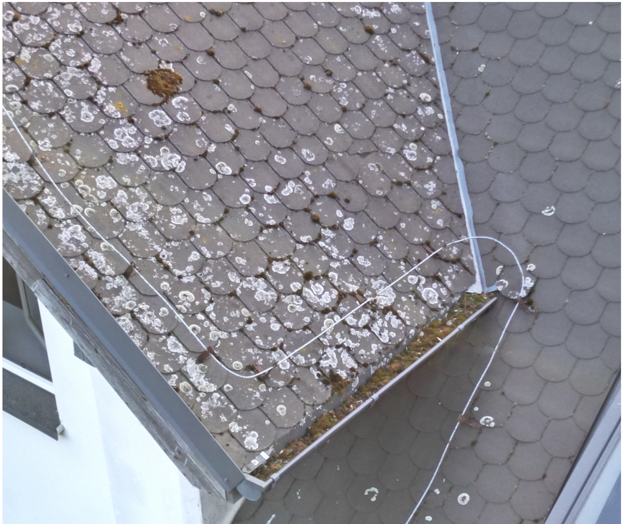
Photo 02. Organic material at the roof junction and a cable or line of unconfirmed function.
