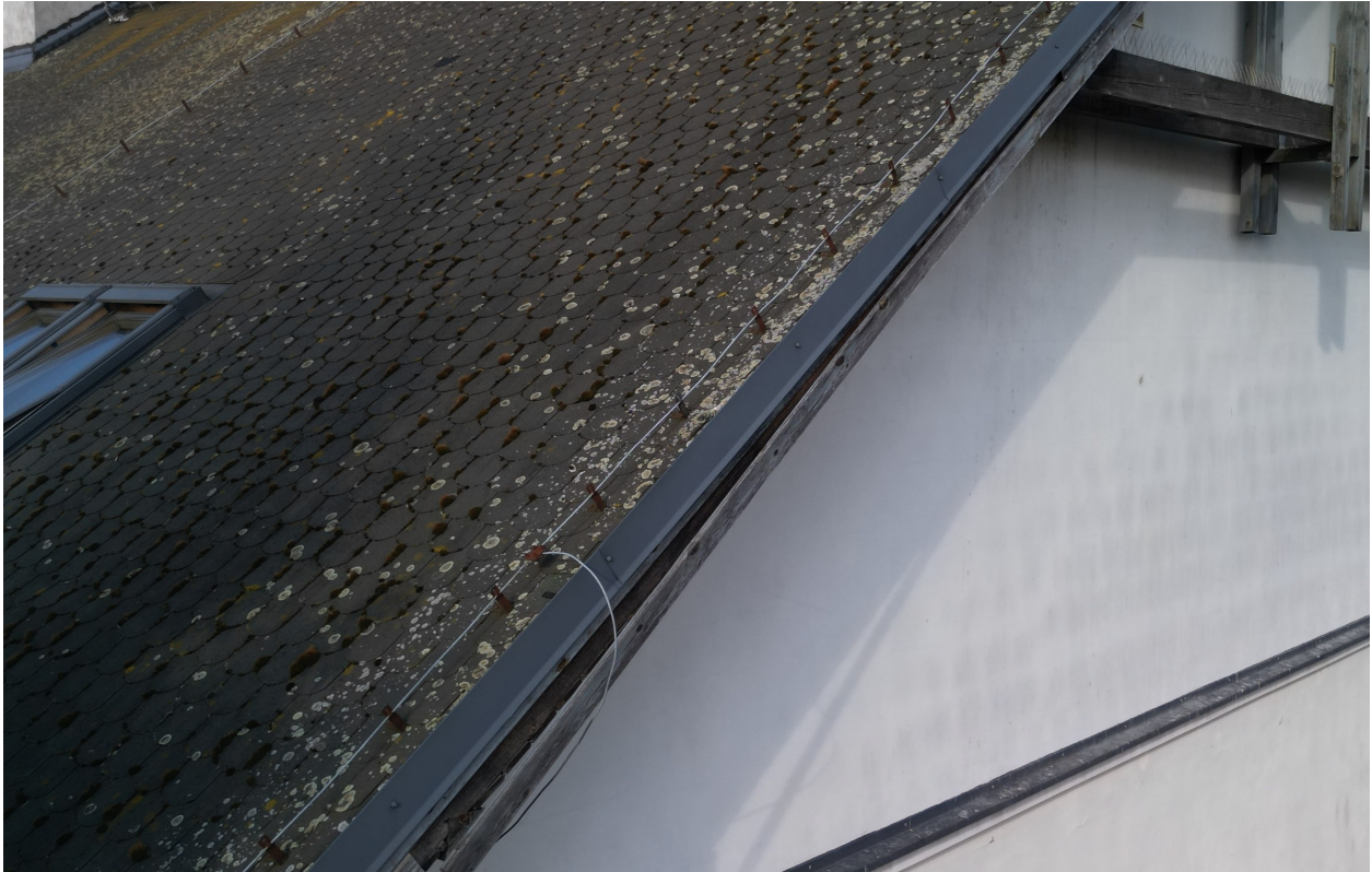
Photo 01. Extensive deposits, moss-like accumulations, visible cables or lines and weathered timber.
