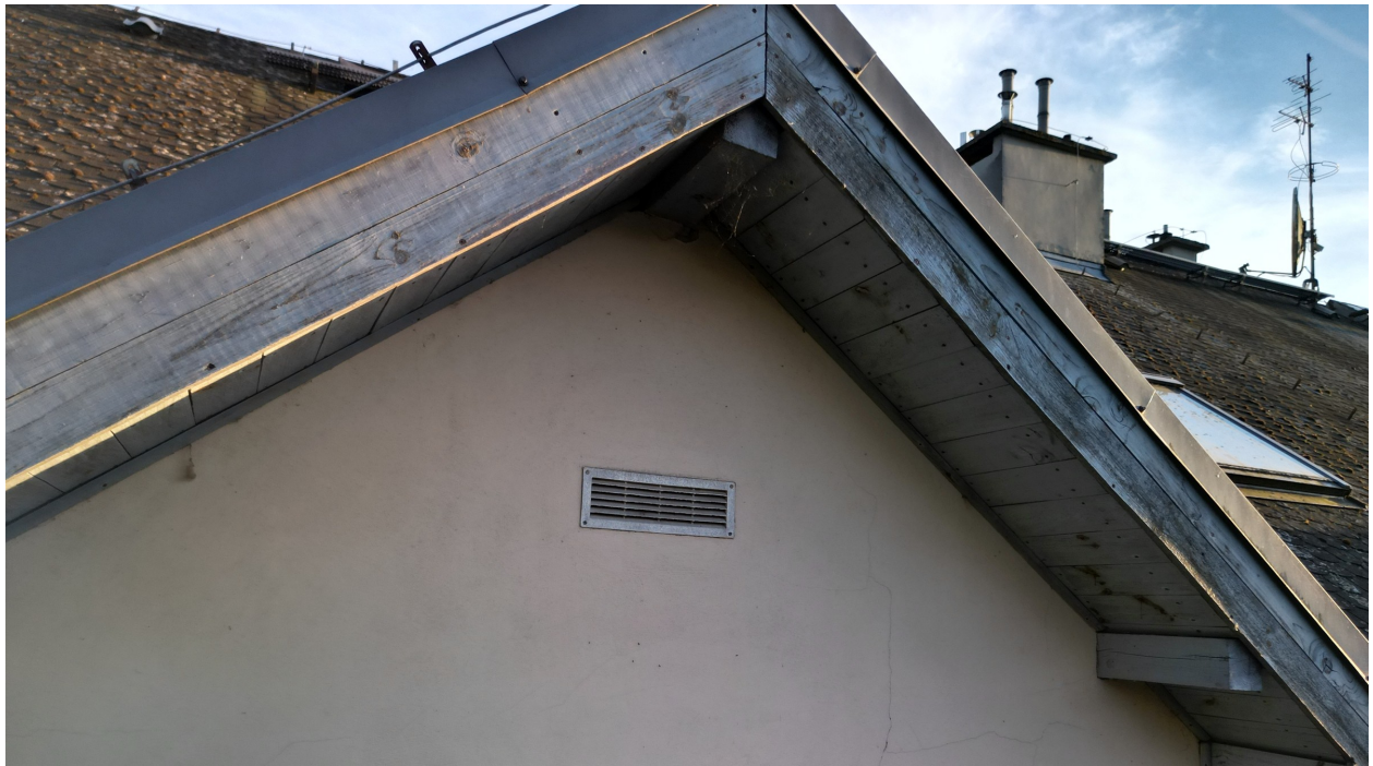
Photo 06. Fine cracks in the render and surface weathering of timber.
